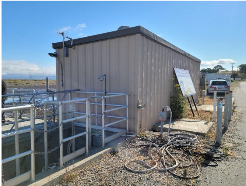
FERRF Pump Station
